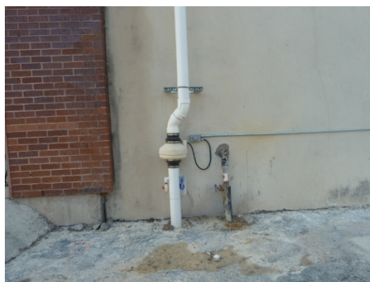
Figure 7. Part of vapor mitigation system installed at Savings Square Shopping Center. It has been operating since March 2009.
