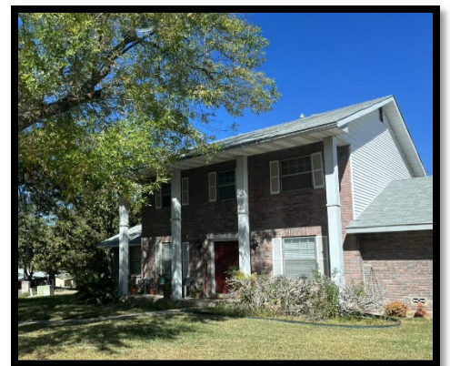
Figure C. Home with dead vegetation in the 5-15’ HIZ and next to wooden columns, increasing fire risk.
