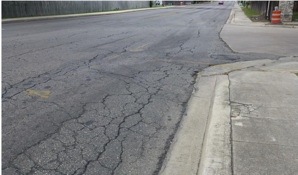
Illustration of typical street condition along Evers Rd.
